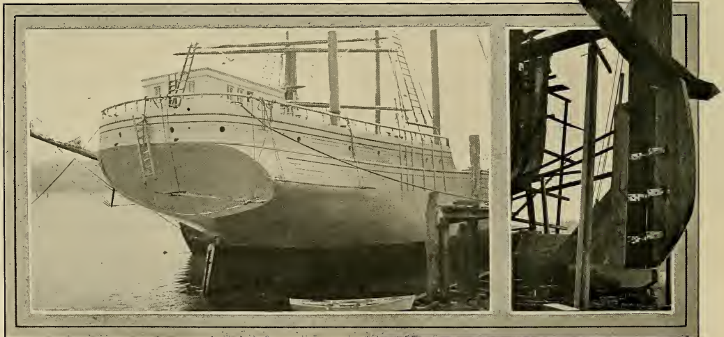
FIG. 101—FINISHING TRANSOM STERN ON A 5-MASTED MOTOR SCHOONER. FIG. 102—DETAIL OF RUDDER AND RUDDERPOST ASSEMBLY
