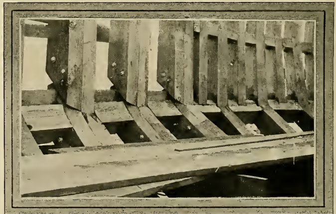
FIG. 130—ARRANGEMENT OF TIMBERS INSIDE THE SAME STERN AT THE POINT SHOWN IN FIG. 129
