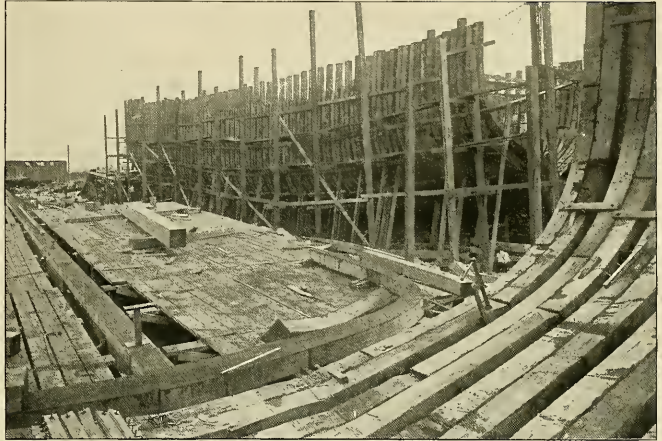
FIG. 50—FRAMING STAGE LAID ALONGSIDE KEEL—THE FRAMES ARE HOISTED INTO POSITION BY MEANS OF A SIMPLE TACKLE
