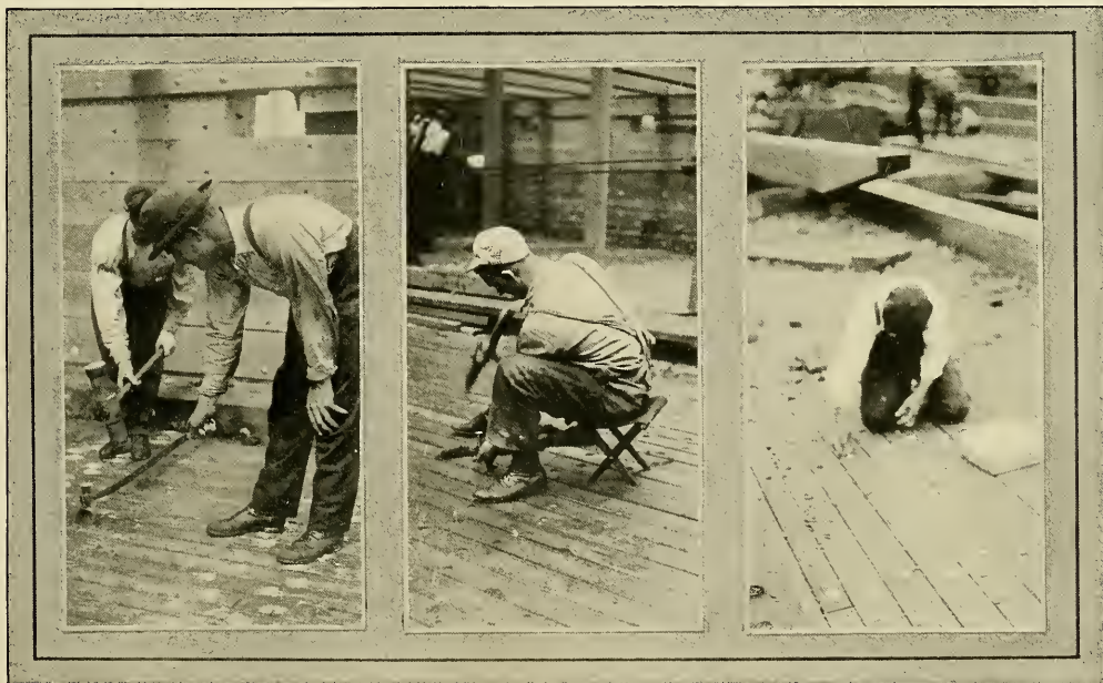
FIG. 177—CAULKING DECK USING HEAVY MAUL. FIG. 178—FINISH CAULKING. FIG. 179—INSERTING PINE PLUGS OVER SPIKEHEADS IN DECK
